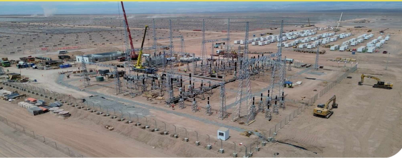
As an investor in solar and battery storage in Chile, MetLife is helping advance the country's clean energy transition.
